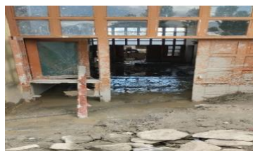
Figure 5 DJ High School damaged by flood
