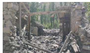
Figure 6 Houses damaged by flood
